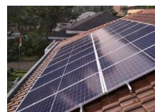
Solar Power Plants
