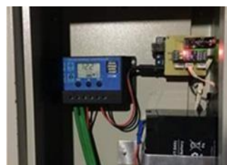
Weather monitoring components
